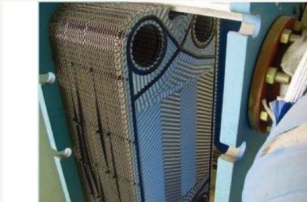
Plate heat exchanger
